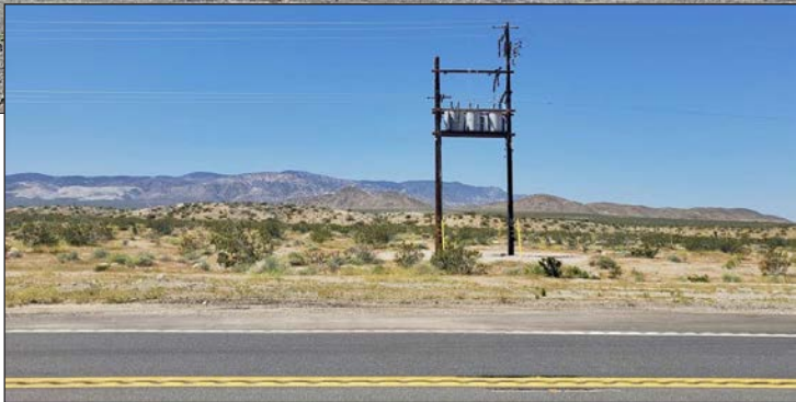
PM 31.3W - Scenic View with Intrusion: A transformer on the west side of the highway, seen from PM 31.3 looking west.
